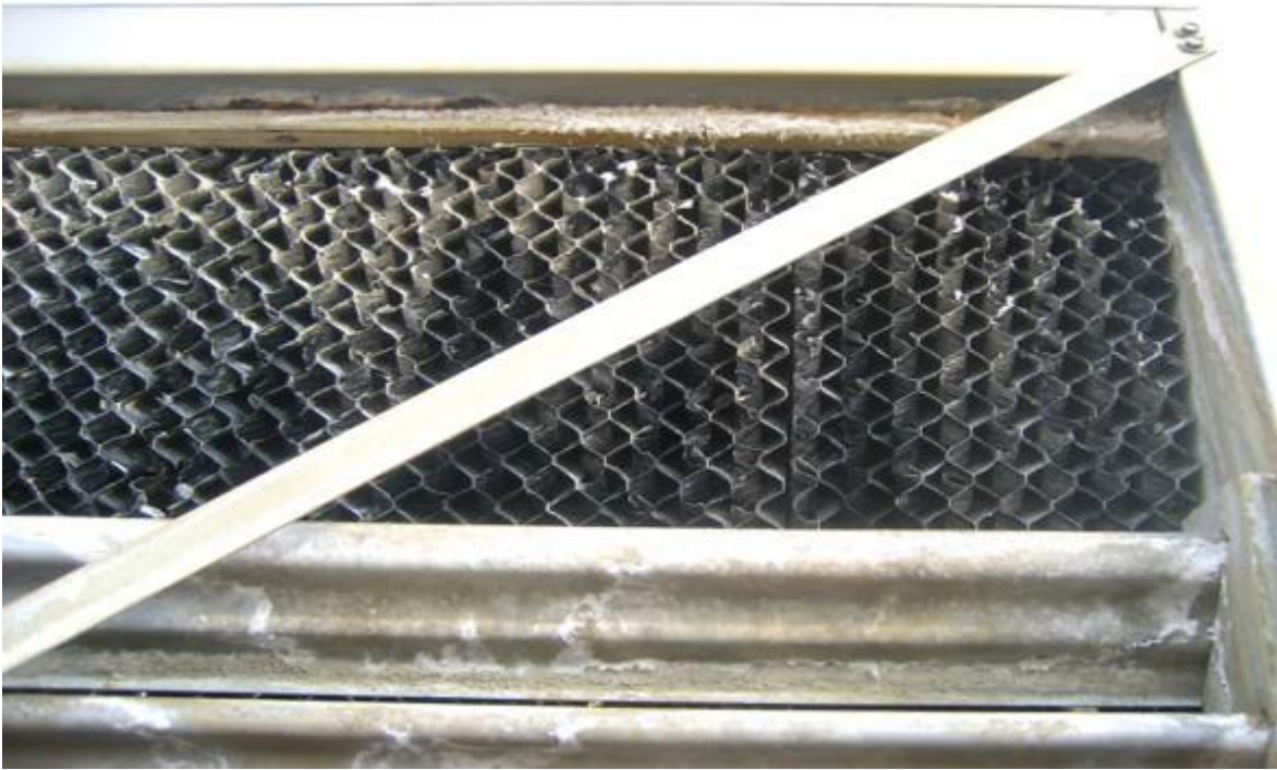
Cooling tower media from 16 year old phase one test facility before starting on ProMoss™
