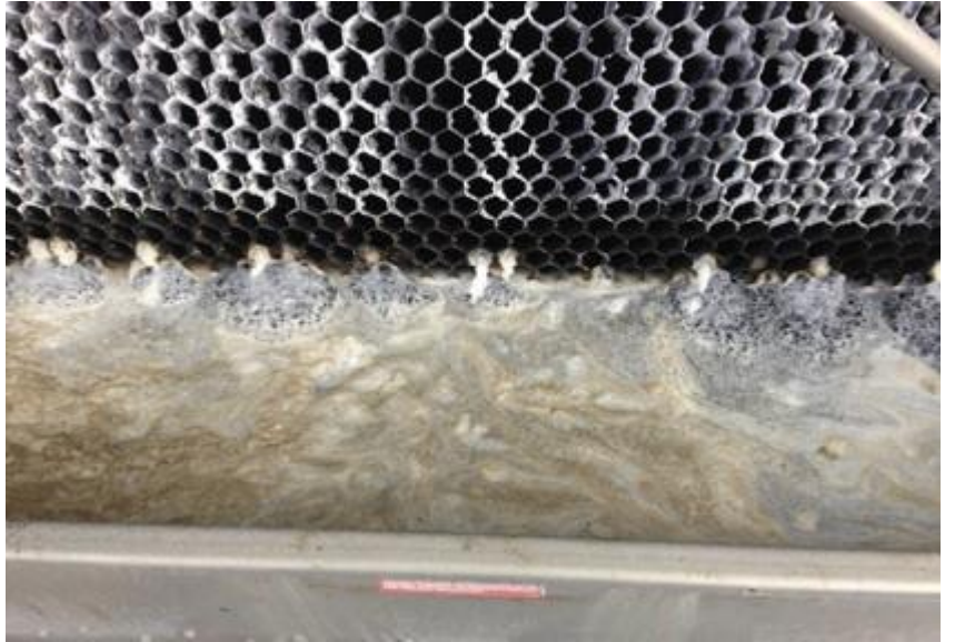
Foaming in return water (note foam coming from the media)
